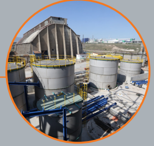
Stok Tank Storage Tank
