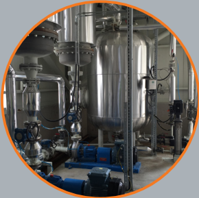
Proses Tank Process Tank
